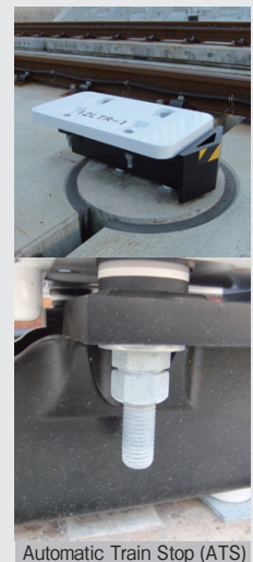
Automatic Train Stop (ATS)
