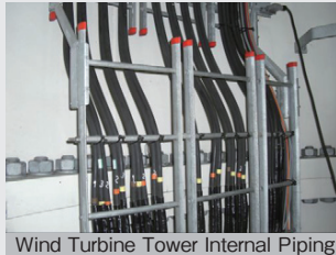
Wind Turbine Tower Internal Piping
