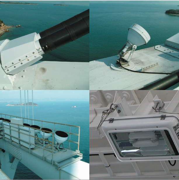
Long-span Bridge Ancillary Equipment Joint
