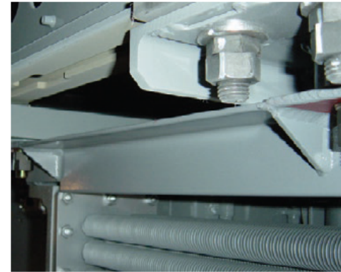
Shinkansen underfloor devices
